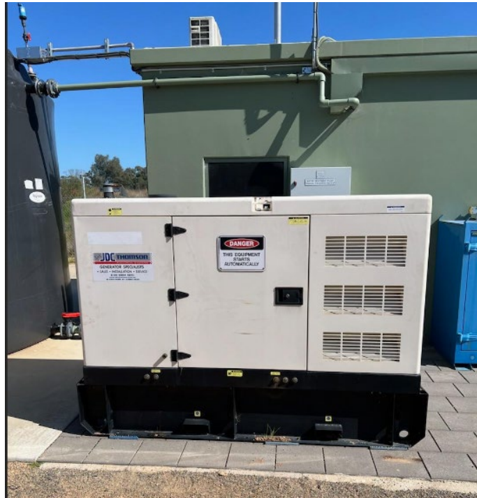
Figure 3: New electrical generator installed at the Tomingley Water Treatment Plant
